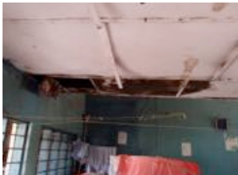
Damaged sealing in Landry section
