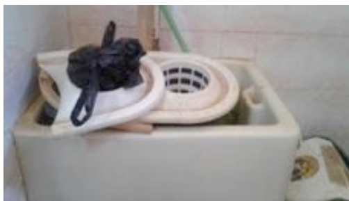
Disorganized sluice room
