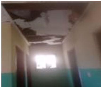
Damaged sealing in a ward
