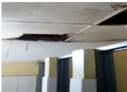
Damaged sealing in the toilet
