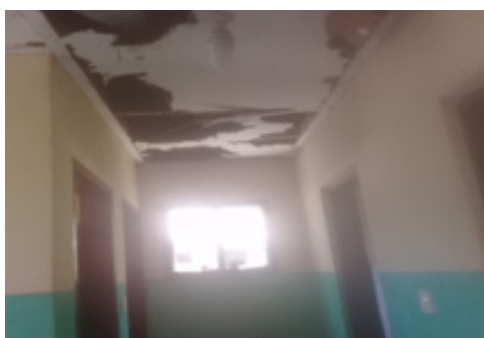
Damaged sealing in a ward
