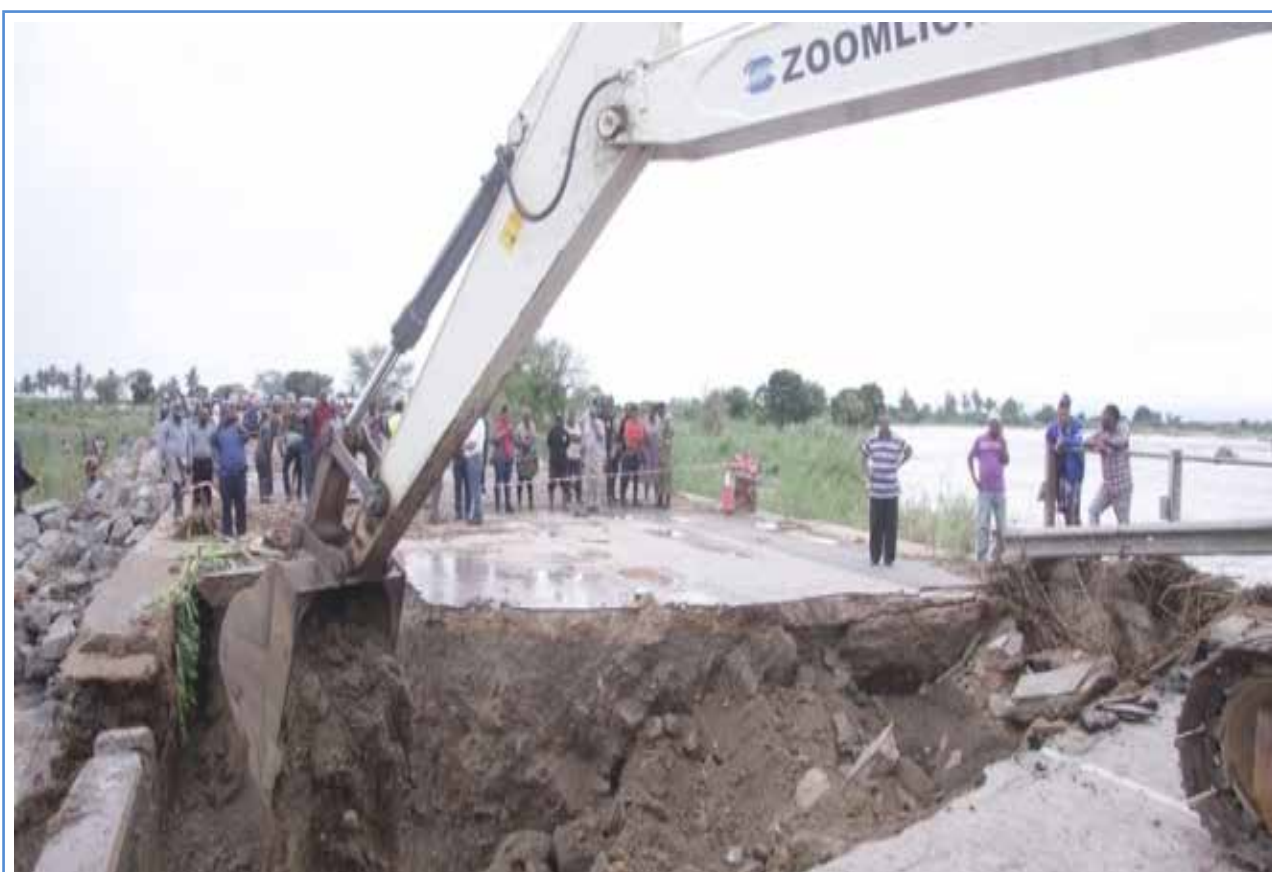
Figure 127: Road and bridge damage by floods at Dumila, Morogoro region
