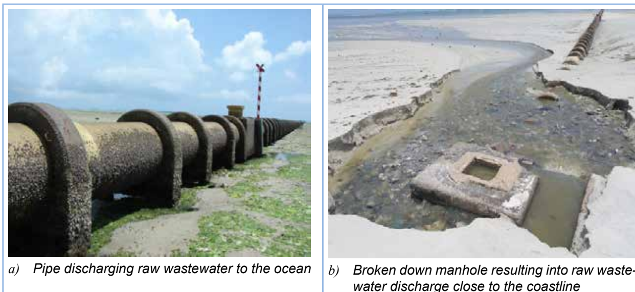
Figure 1010: Dar es Salaam wastewater sea outfall
